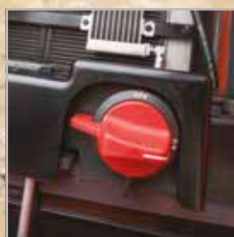
Battery cut-off switch
